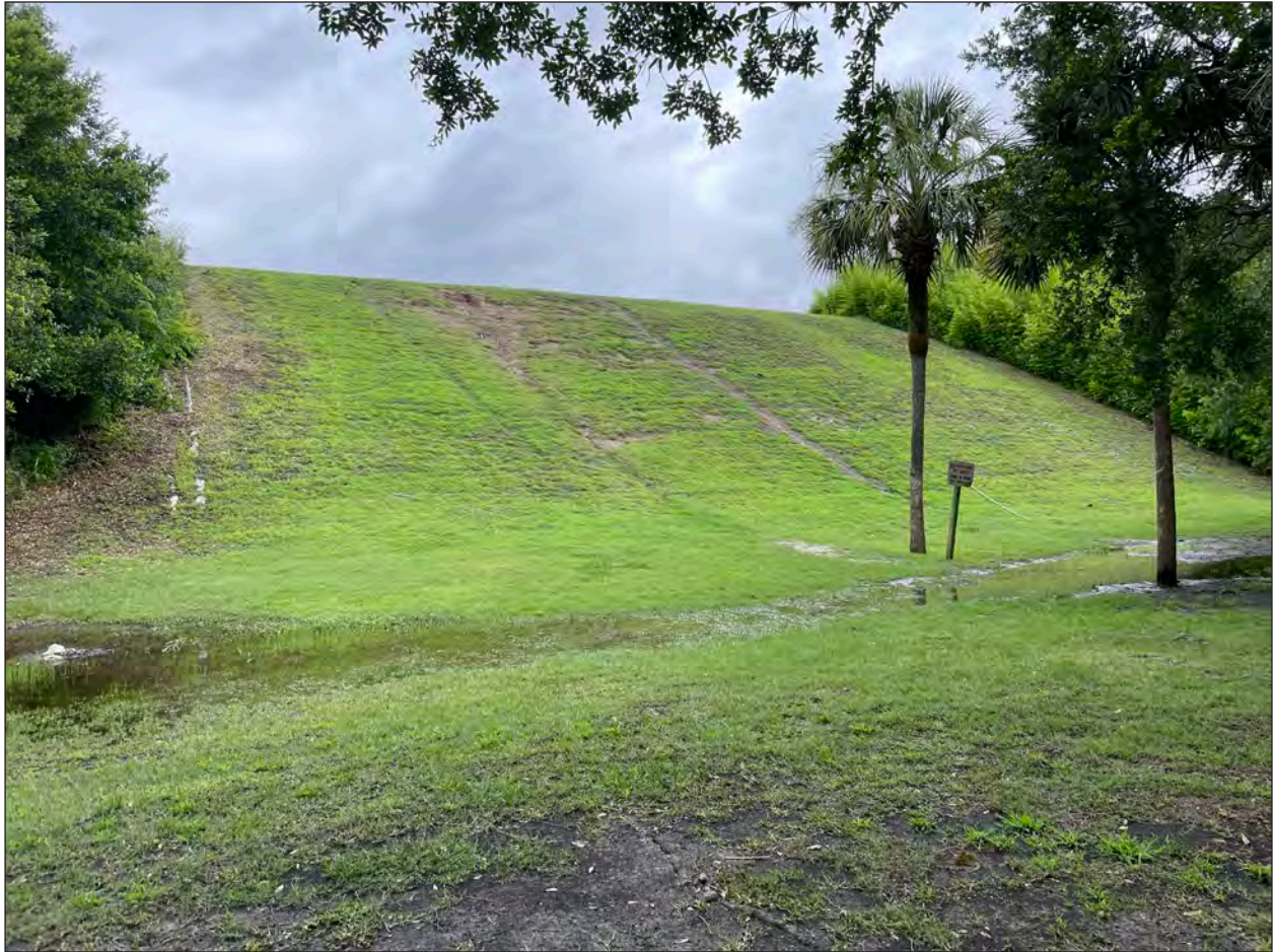
Figure 41. Erosion Gullies and Footpaths in Seaward Face of Battery Butler/Capron
