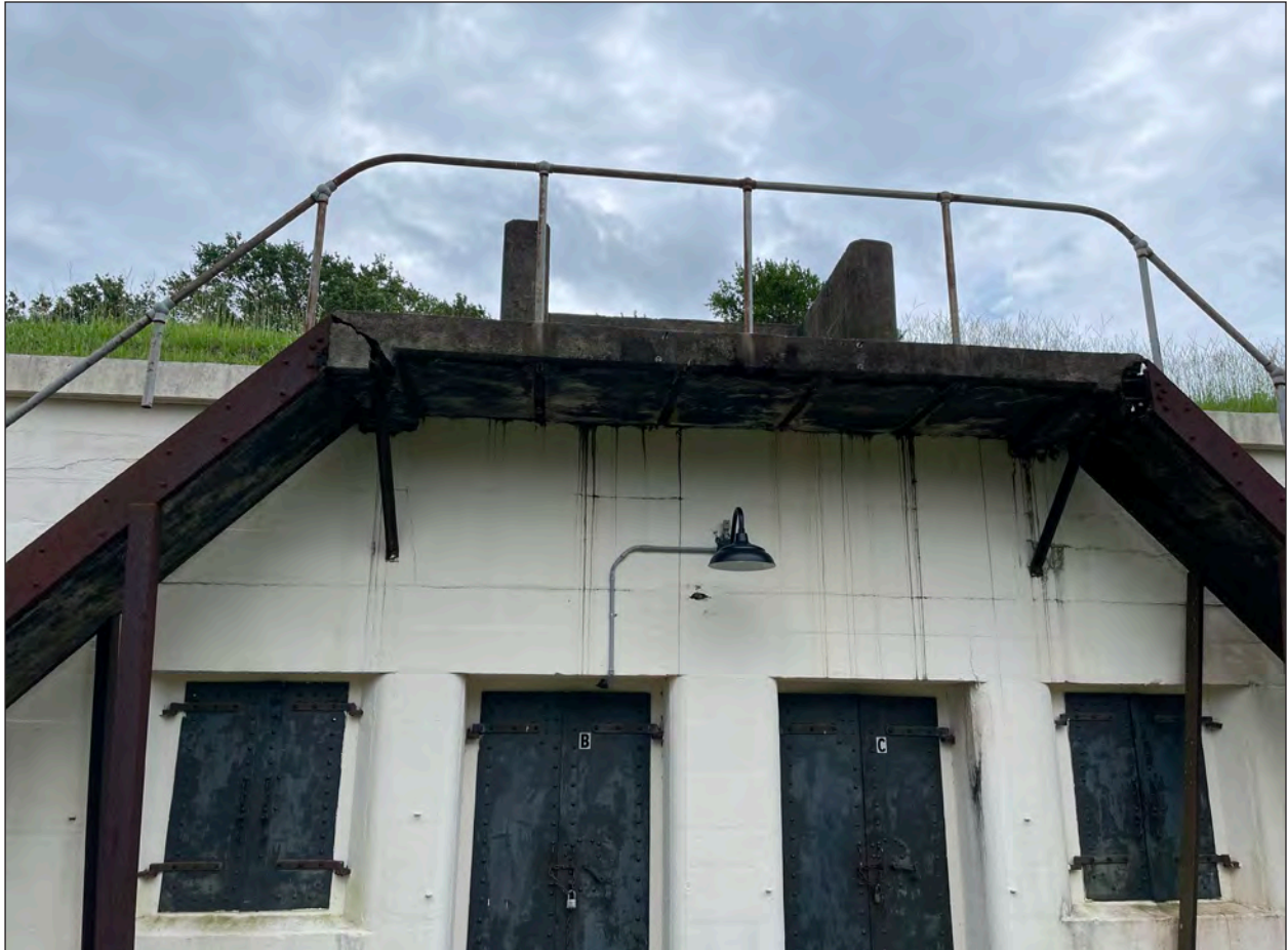
Figure 38. Stairway with Cracked Concrete and Twisted Metal Frame
