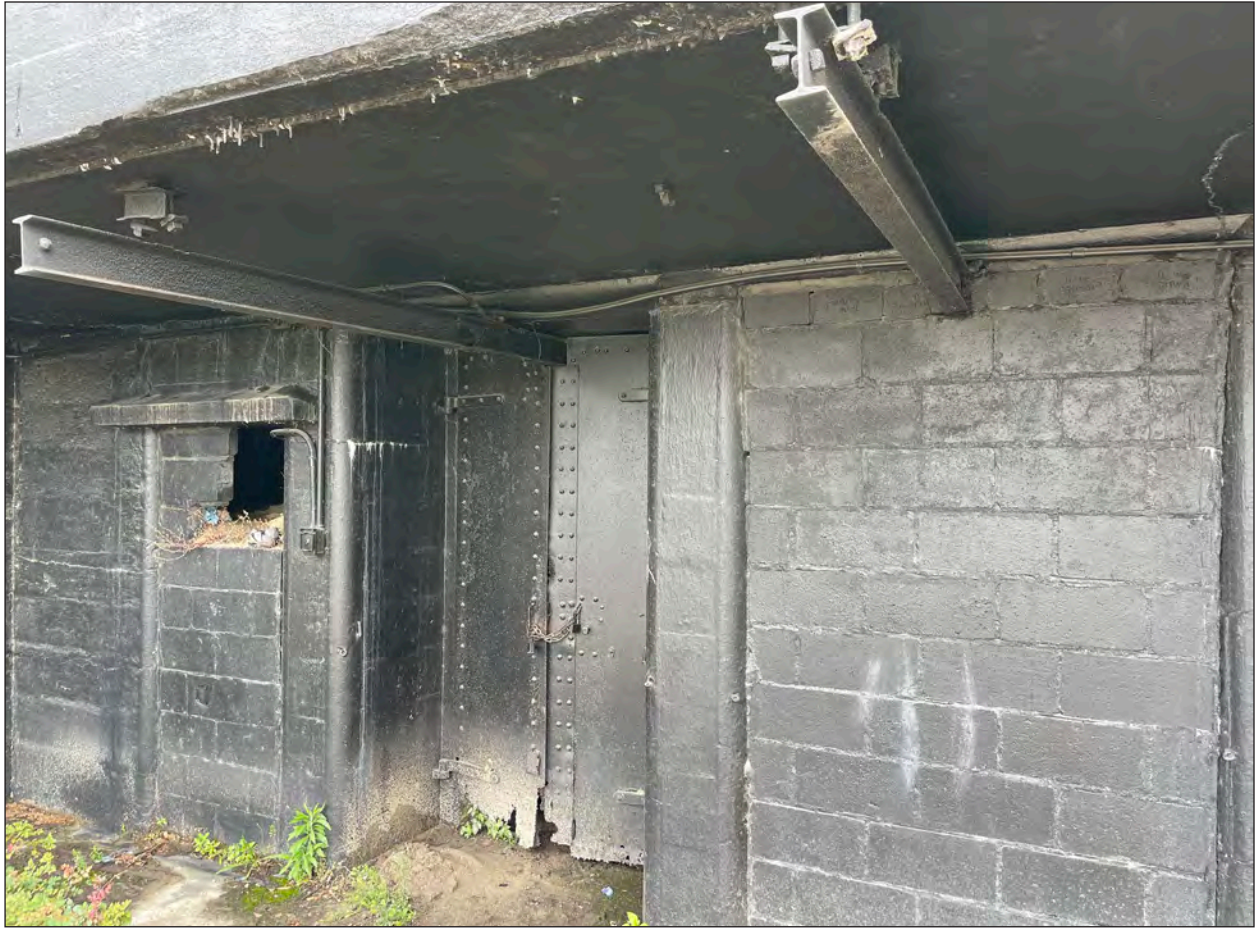
Figure 39. Detached I-Beam and Doorway Infilled with CMUs
