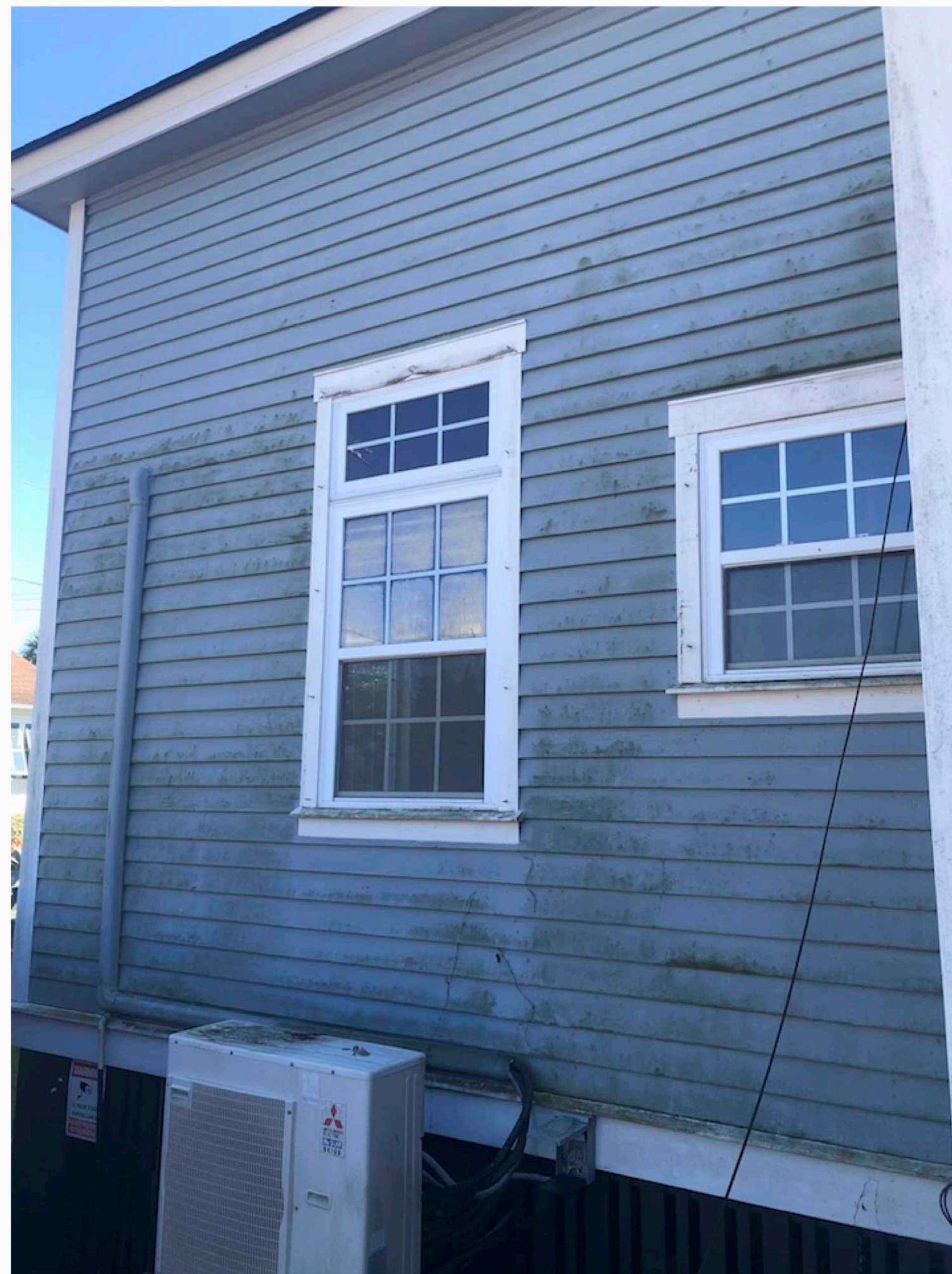
NONHISTORIC VINYL WINDOWS, TYP. *note the simulated muntins/grilles: located between insulated glass
