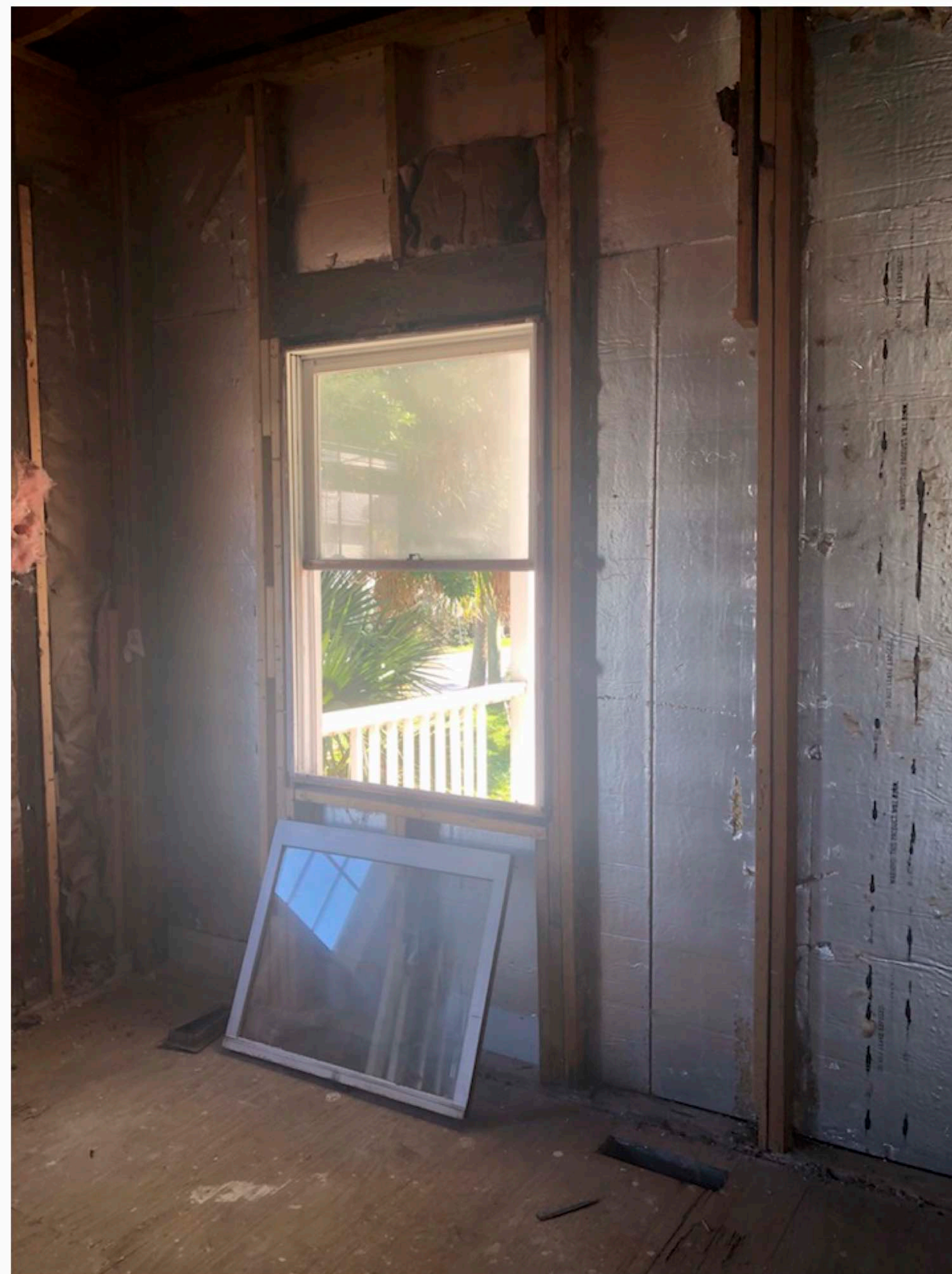
NONHISTORIC VINYL WINDOWS @ FRONT (ION AVENUE)
