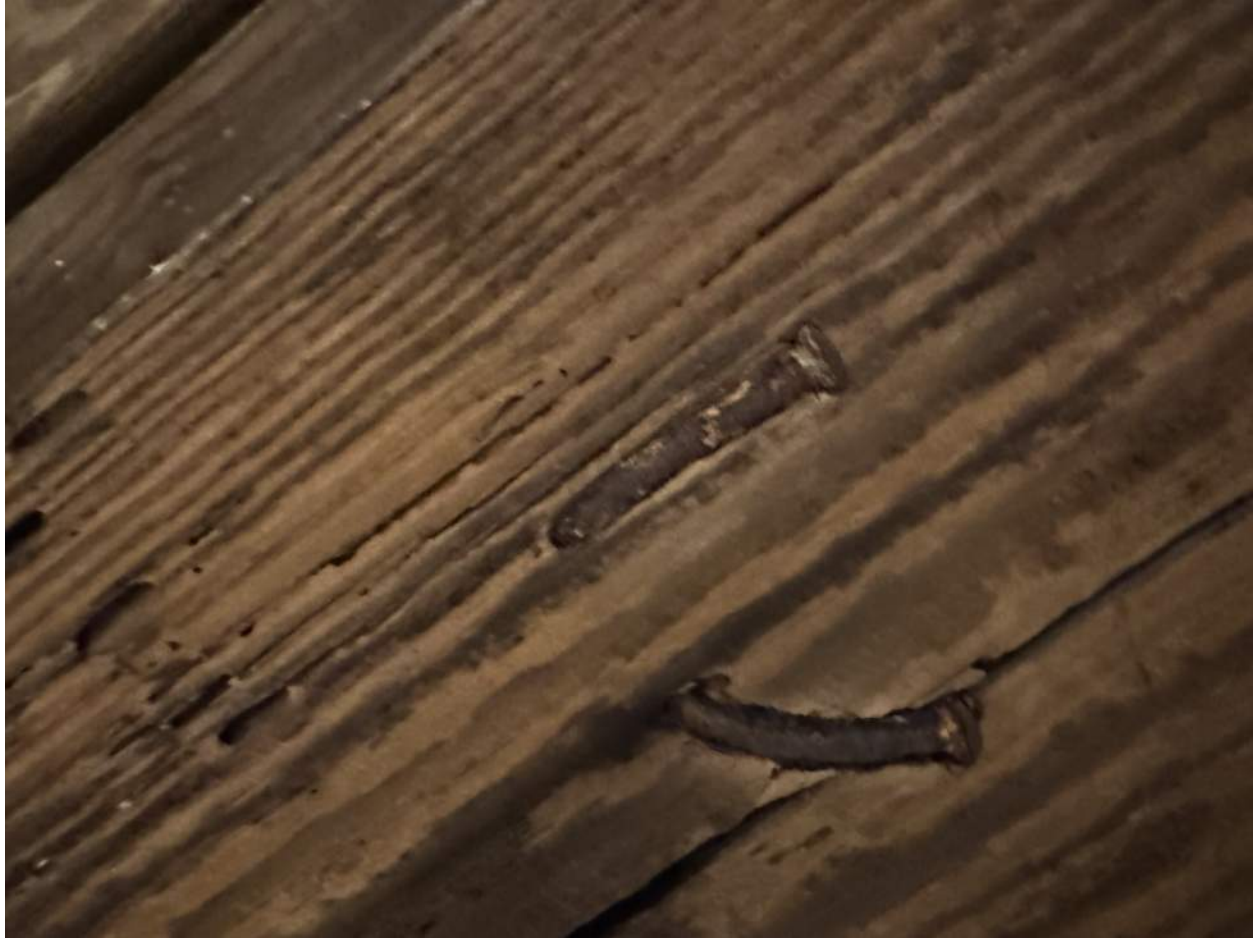
Nails in first floor joists.
