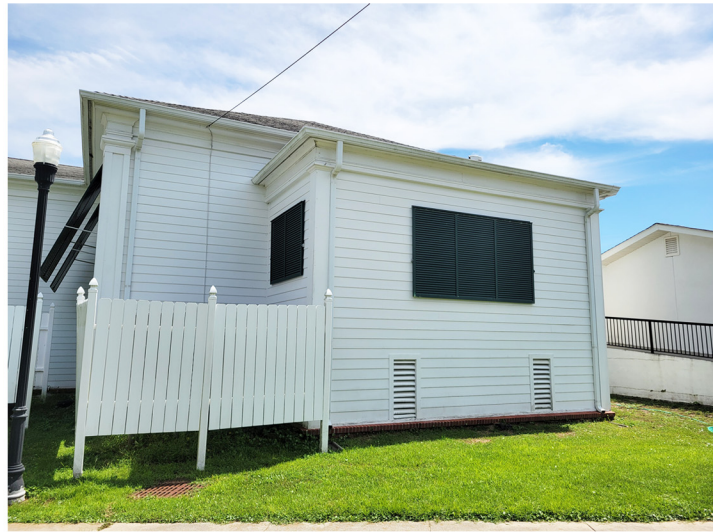
The west end of the building lost all of its original windows.
