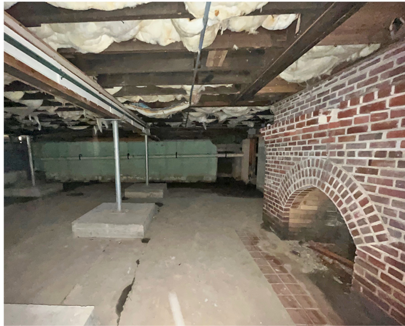
Brick caretaker's fireplace and more recent structural reinforcing.
