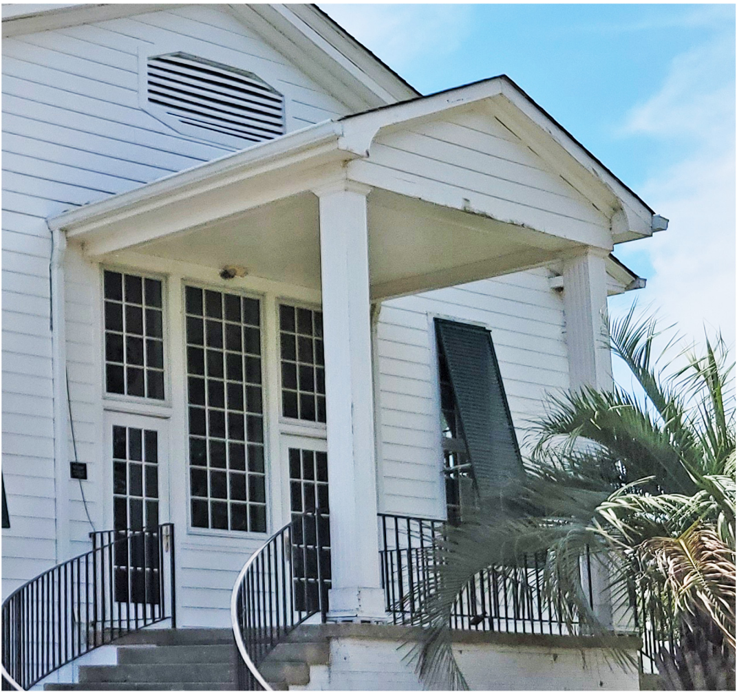
Hollow metal columns, “pork chop” eave ends, and a general low level of detail on the new portico.
