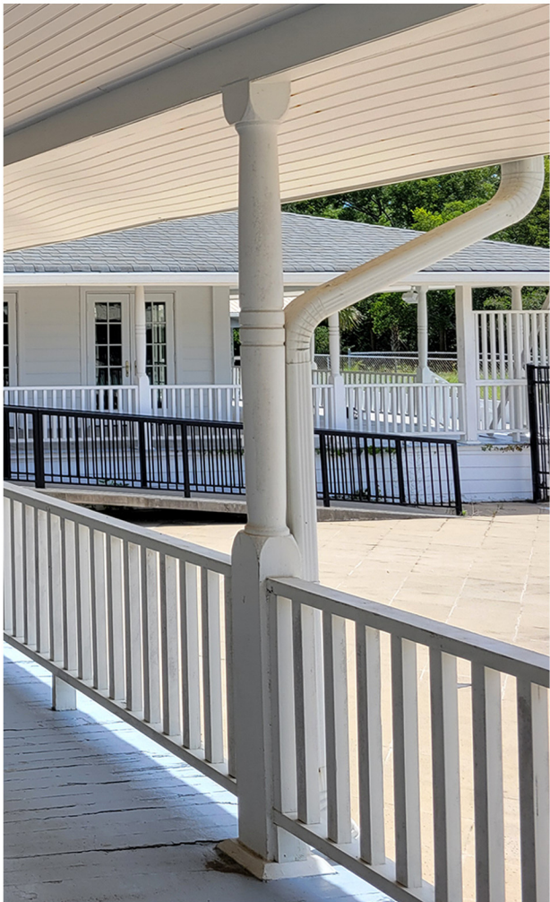
Mid-century round Colonial columns are not compatible wit the Island Beach Cottage style typical of the area.
