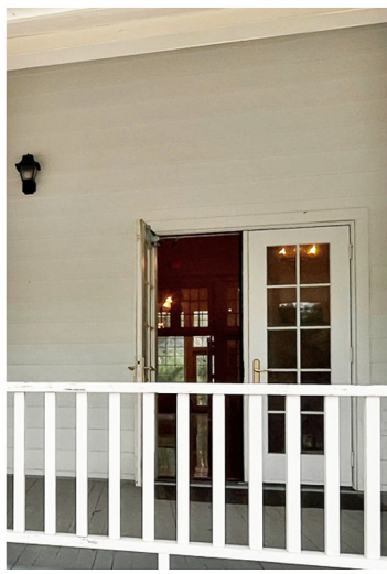
All of the windows above doors were closed in.
