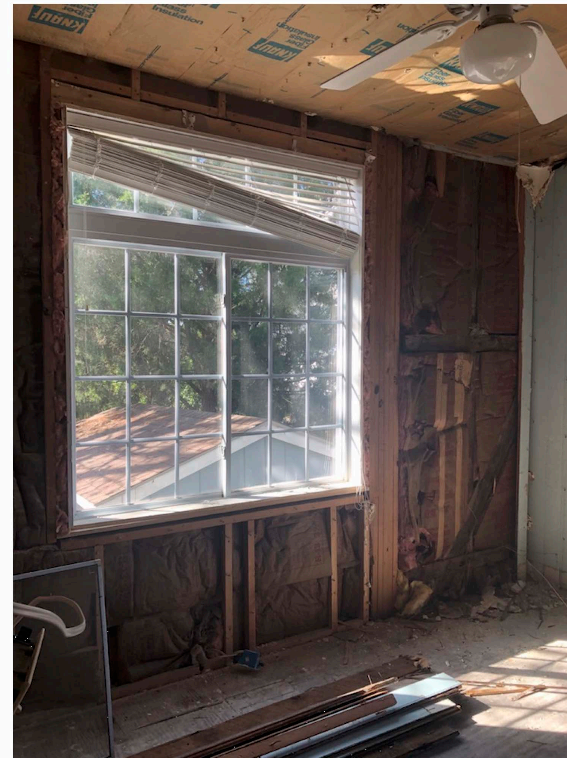
NONHISTORIC VINYL WINDOWS @ SIDE (STATION 22 STREET)
