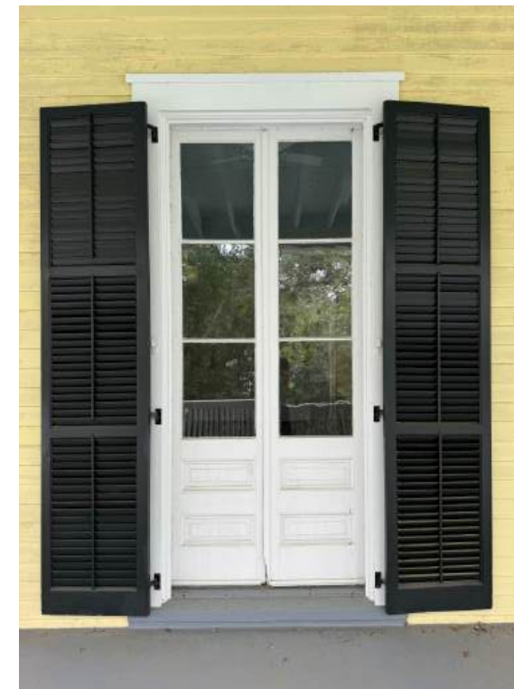
TYPICAL ORIGINAL WOOD AND GLASS FRENCH DOORS DOORS AND LOUVERED WOOD SHUTTERS TO BE REPAIRED AS NEEDED
