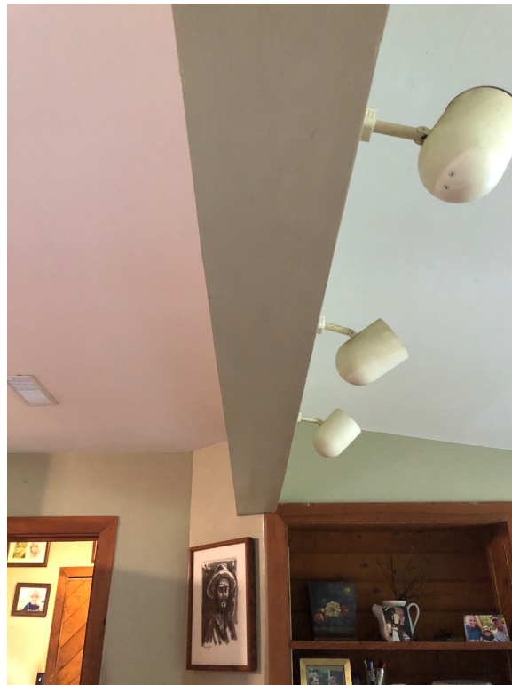
The kitchen extension, constructed in 1992, as seen from the kitchen, looking north. The sheetrock covered lintel with uplighting indicates the original exterior rear wall of the house.
