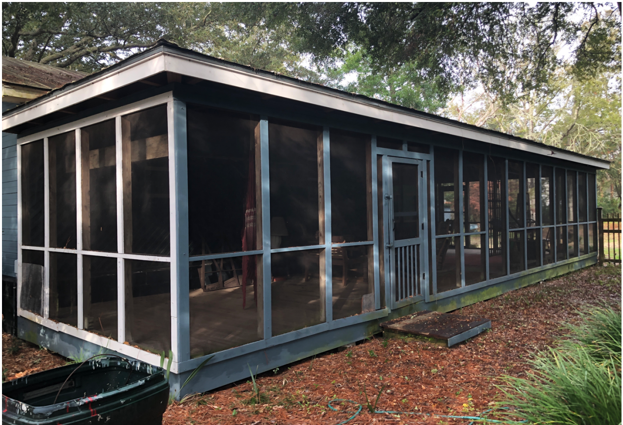
Perspective views of the wrap around side screened porch, which is framed with treated dimensional lumber.
