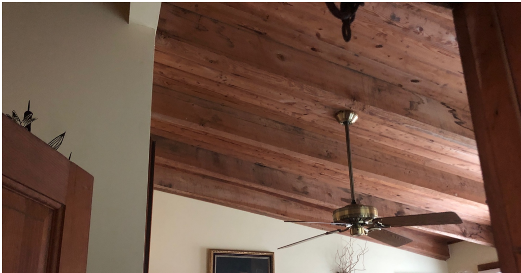
The shed roofed bedroom addition on the rear of the house, the framing of which aligns with the western exterior wall of the ell bay.
