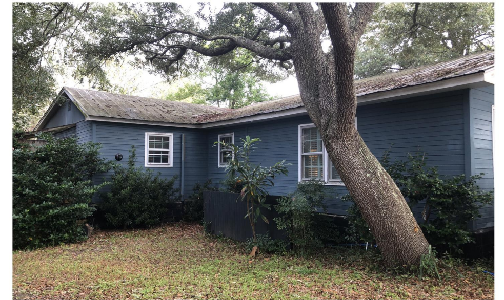
Perspective view of the ell bay, which has vinyl windows and horizontal wood siding.
