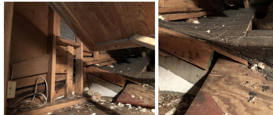
Images the end wall of the house, which has evidence of later repairs. The original back exterior wall of the house can be seen (painted grey and white) and the gable roof over the earlier iteration of the side ell.
