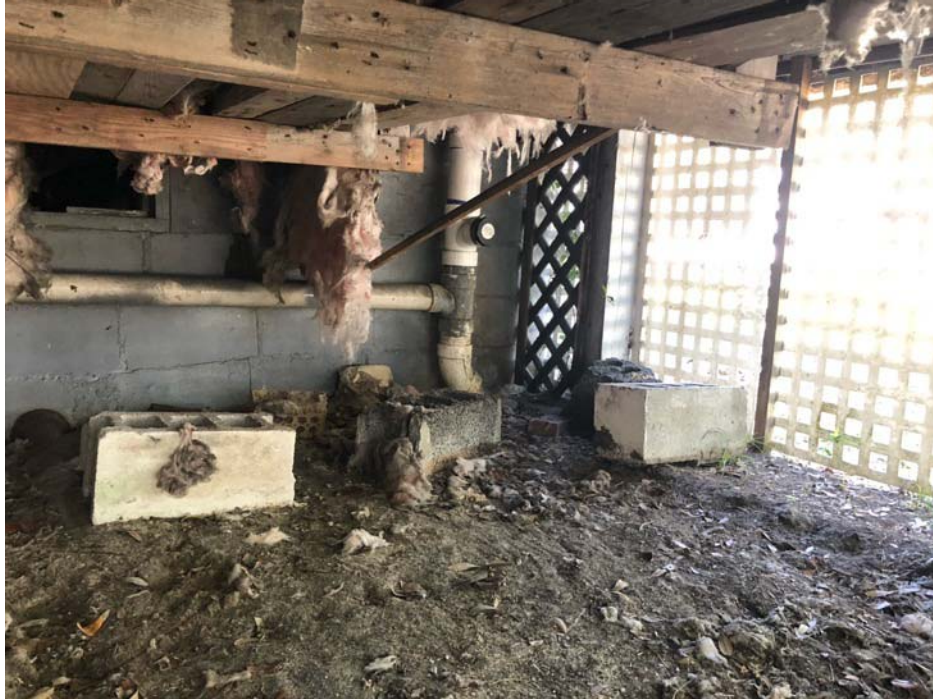
The framing under bay 5 (as viewed looking south from bay 6) shows evidence of deterioration and repairs; part of the joist box is not supported. The photo is taken facing south toward bay 2, the solid CMU wall is the demarcation between the two bays.
