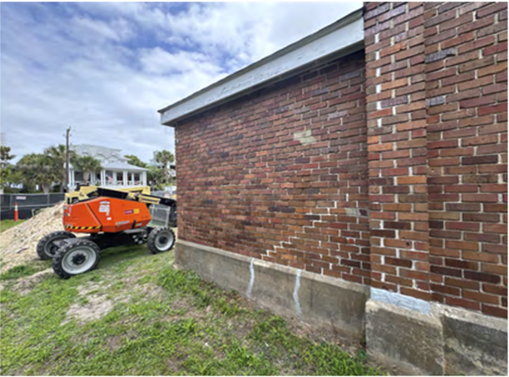
West boiler room exterior. Foundation cracking, and stair-step cracking of brick in multiple places. Previous attempts to patch and re-point.
