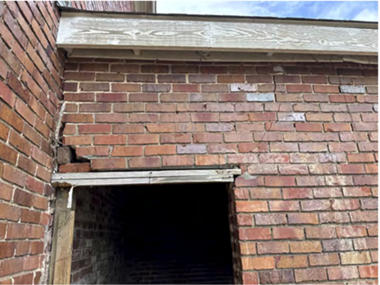
Separation of the boiler room brick from the the main structure and partial collapse.
