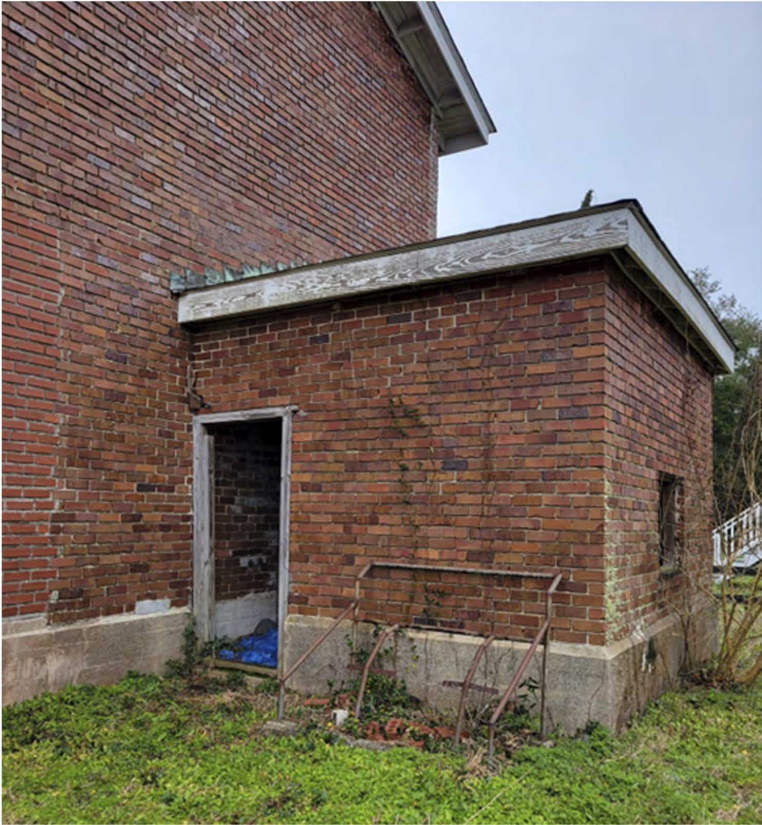
The boiler room has sustained significant damage due to construction defects as well as differential settlement of the main building and the boiler room foundations.
