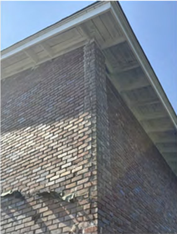
Cracking due to separation continues up the corner of the main structure.
