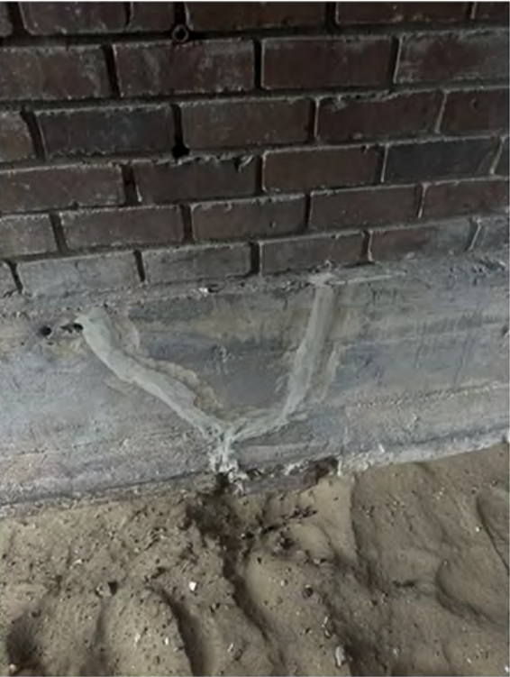
Foundation cracking in boiler room interior.
