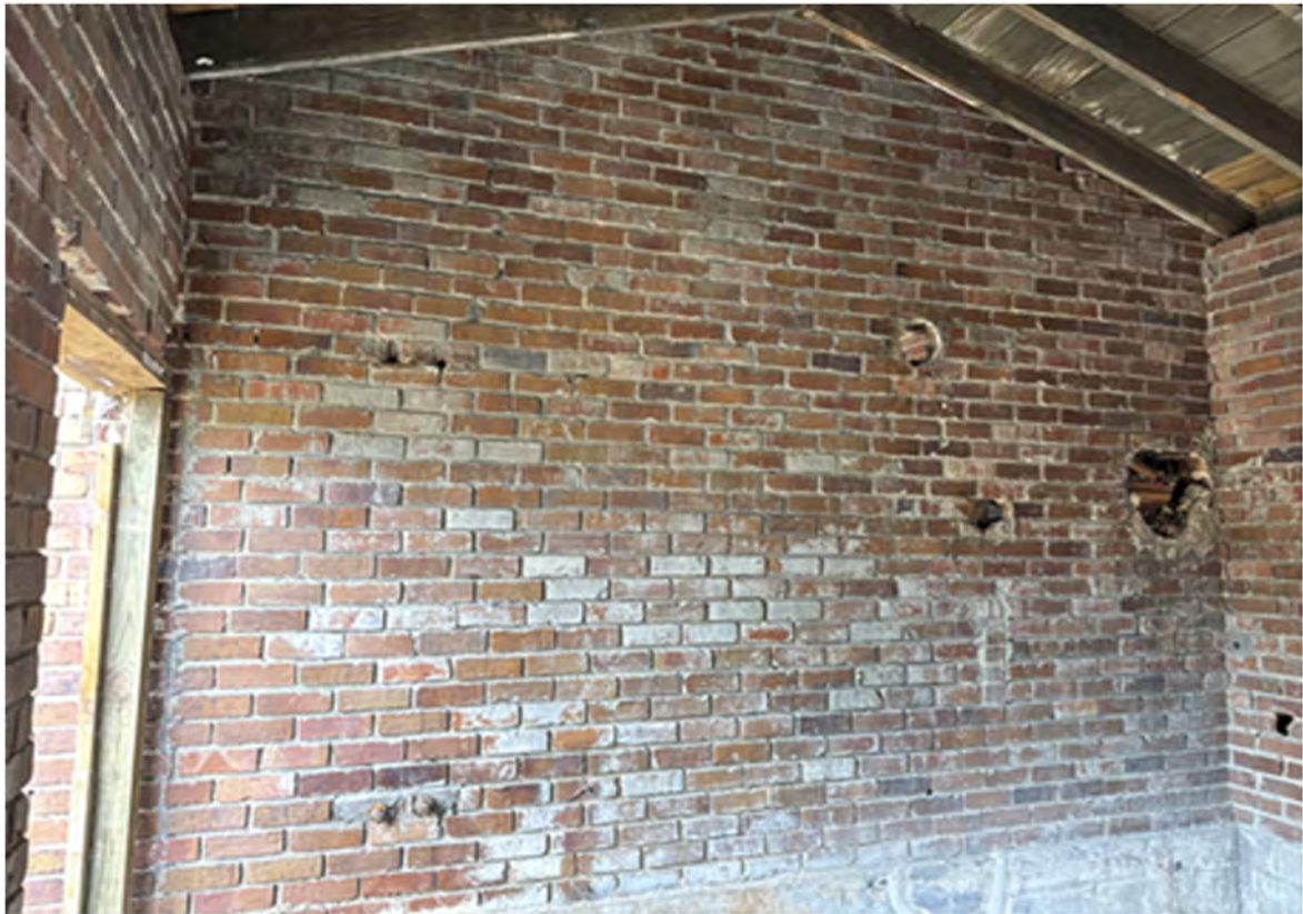
Interior boiler roof, rear wall of main structure. Foundation cracking and separation of walls.
