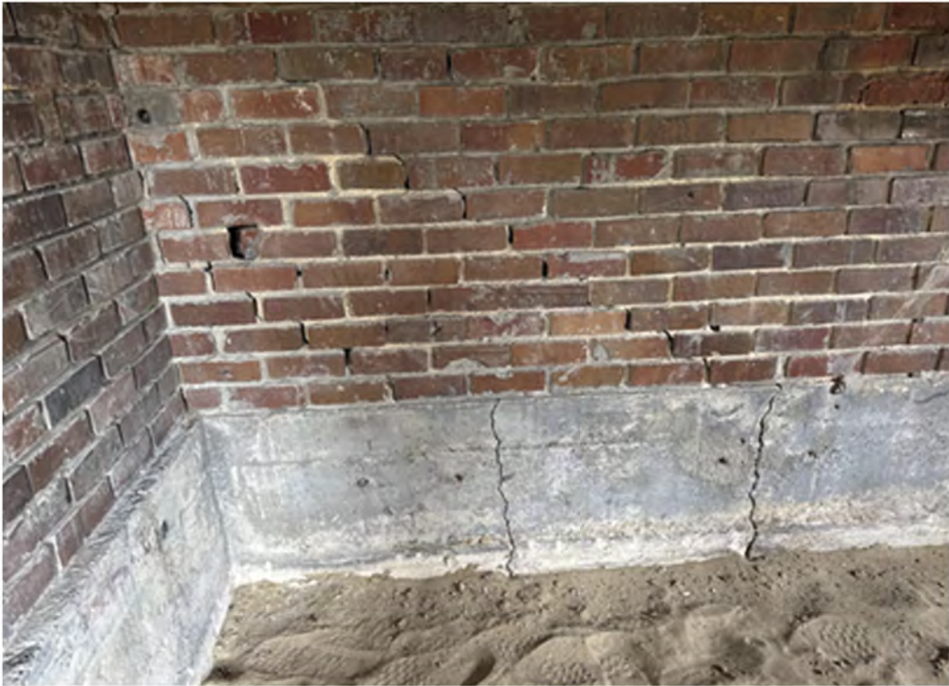
West boiler room wall interior. Foundation cracking, and stair-step cracking of brick in multiple places.
