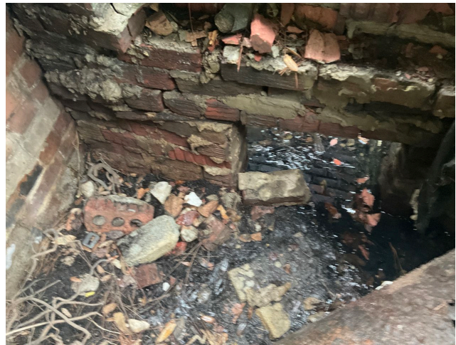
Damaged Inlet Structure
