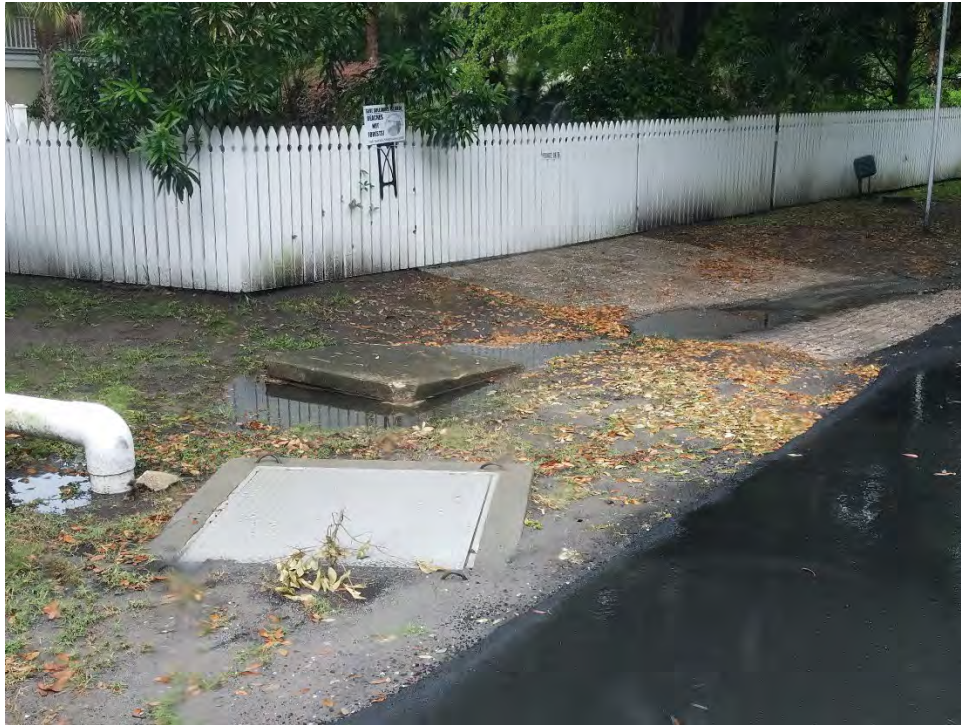
Four days after a rain event (water floods).
