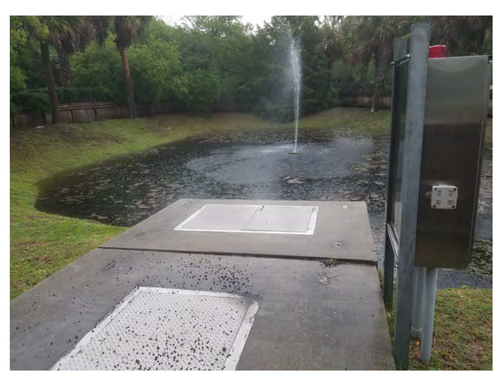
APRIL 2017, ATLANTIC AVENUE AT SCE&G PROPERTY/PUMP STATION DURING AN APPROXIMATE 4.0-INCH RAIN EVENT (2-YEAR STORM EVENT IN CHARLESTON COUNTY ESTIMATED 4.6-INCH IN 24 HOUR)
