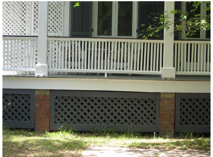
These traditional diagonal lattice panels are appropriately placed between the porch foundation piers at 1744 Iron Avenue.
