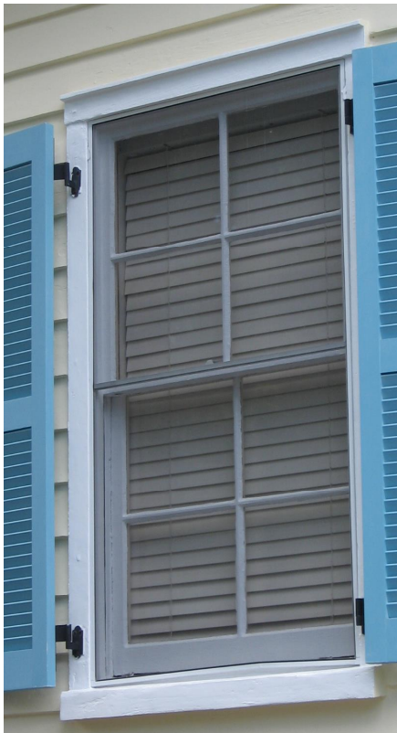
Some of the oldest windows in the districts are four-over-four wood sash design (2424 Middle Street).
