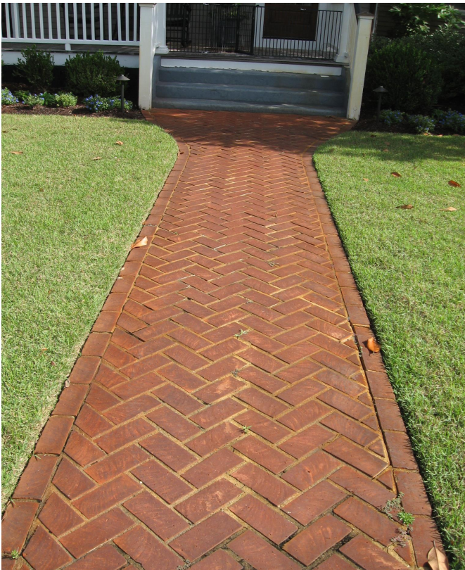
Brick walkways from the early- to -mid-20th century should be preserved and maintained as at 1722 Middle Street.
