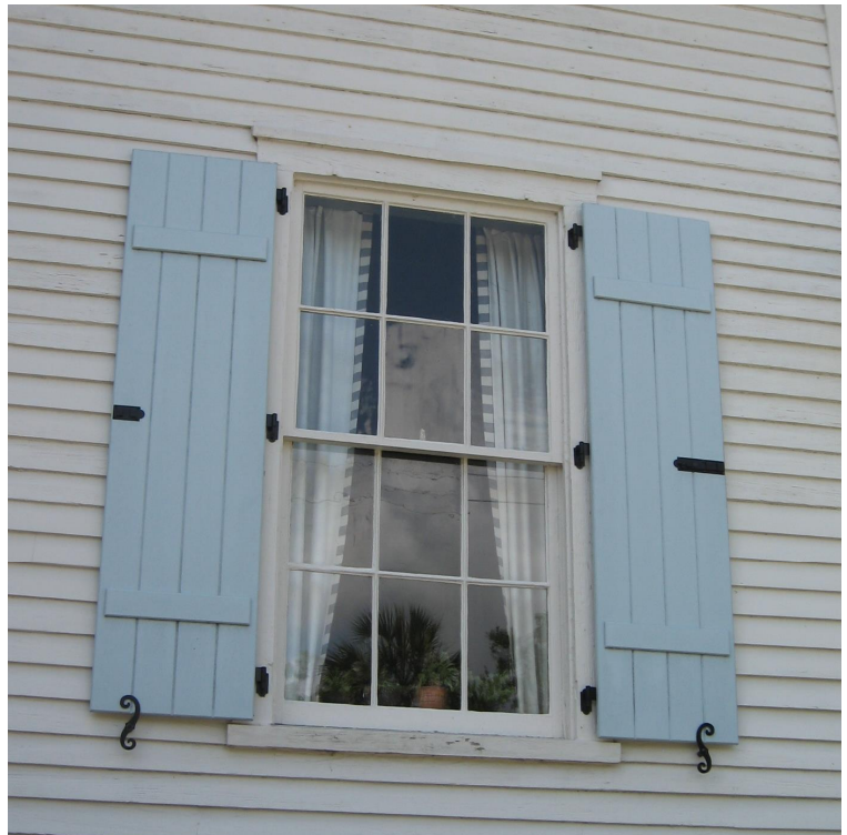
Many appropriate shutter designs are within the historic districts. These vertical board shutters are operable and can be closed to protect the window during storms (312 Station 16 Street).
