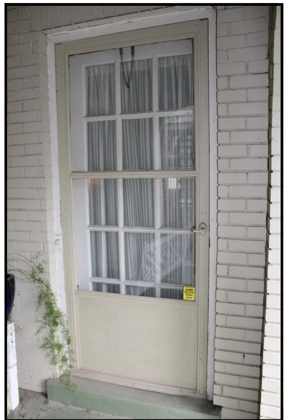
NO: Storm doors should be full-view to allow the historic door to be viewed behind it.
