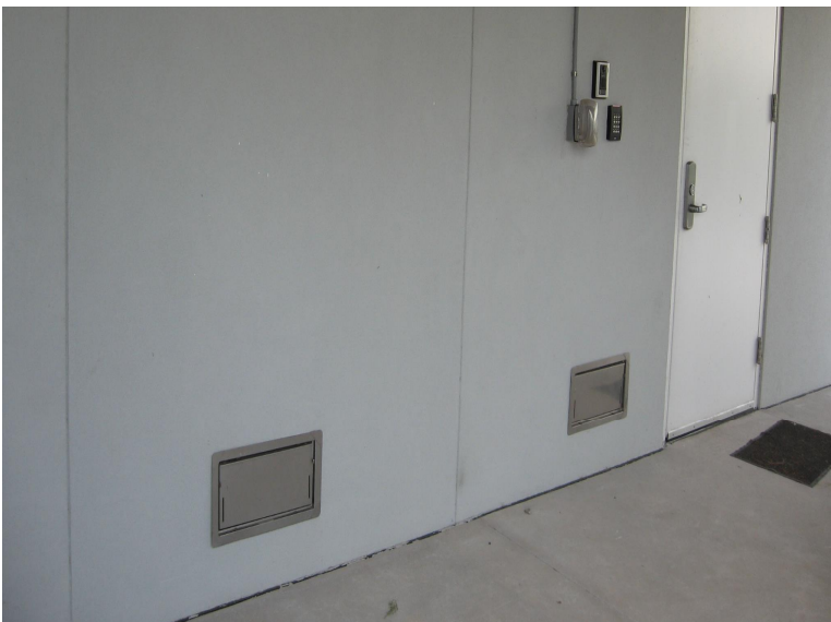
Appropriate design flood vents located at the Town's Fire Station at 2050 Middle Street.
