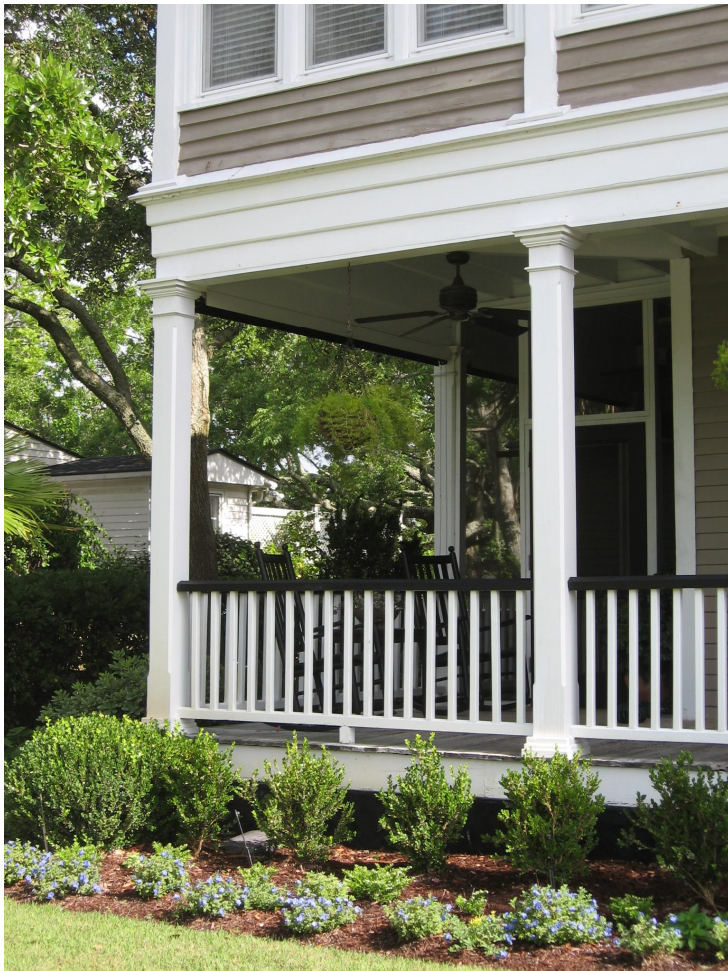
Home owners can familiarize themselves with the principles of appropriate treatment of historic features such as the repair of original chamfered wood columns and balusters (1722 Middle Street).
