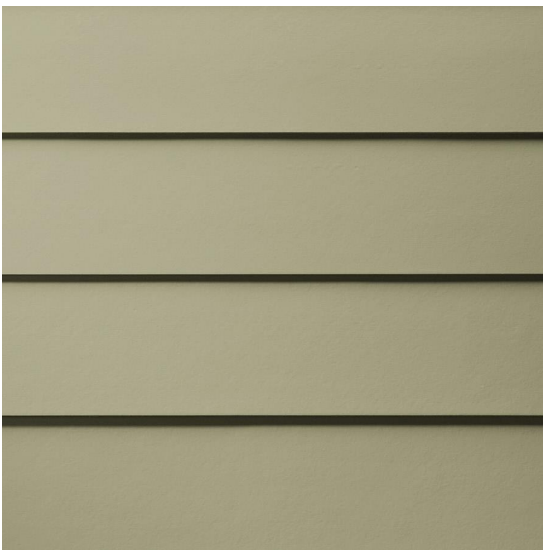
YES. Cementitious siding for should resemble historic wood siding as closely as possible in width and reveal.
