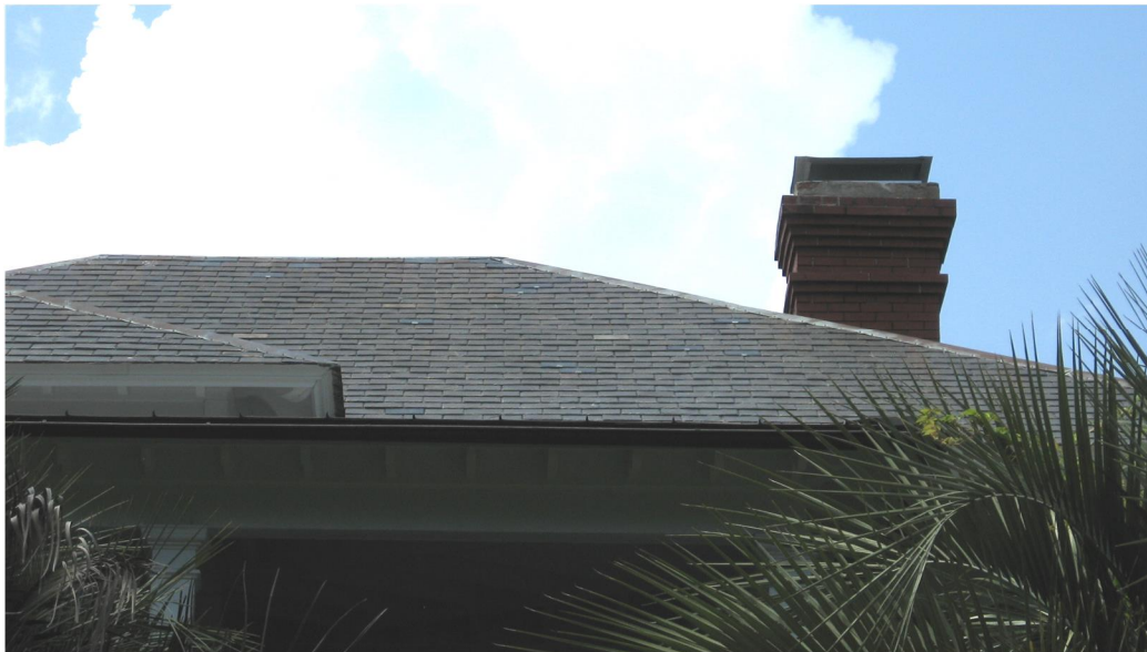
Only a few original slate roofs exist in the historic districts. These can last indefinitely and are important defining features of a property (1760 I'on Avenue).
