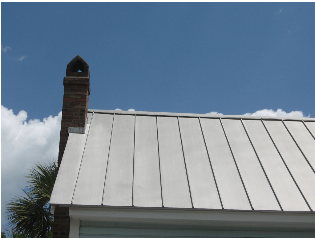
The installation of standing seam or crimped metal roofs is appropriate as long as they consistent with traditional seam patterns and spacing (1002A Middle Street).
