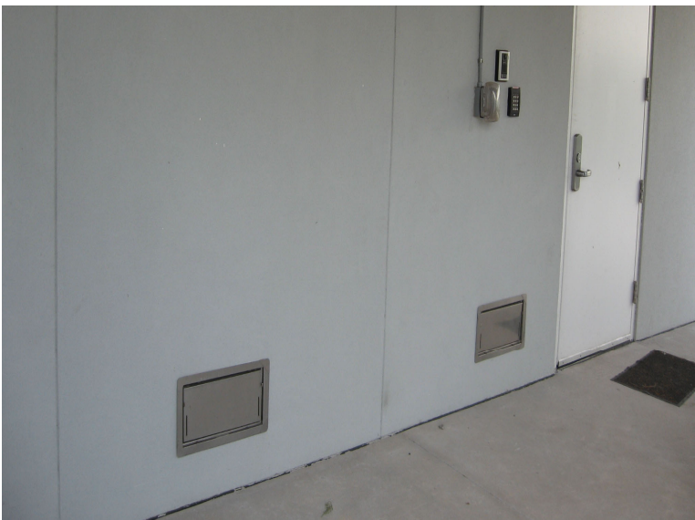
Appropriate design flood vents located at the Town's Fire Station at 2050 Middle Street.
