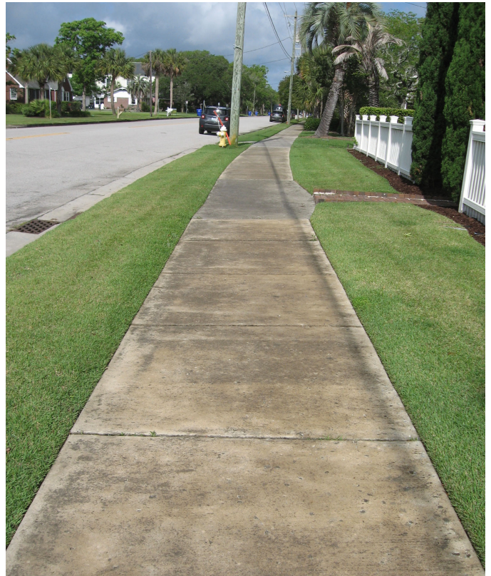
Concrete sidewalks added in the early- to -mid-20th century should be preserved and maintained as in the 1700 block of Middle Street.
