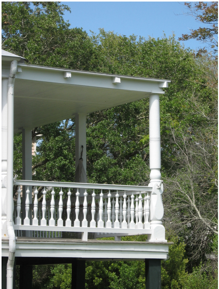
Milled wood porch columns and turned balusters on the porch railings are one of the most important defining features of a dwelling's style (1112 Osceola Avenue).
