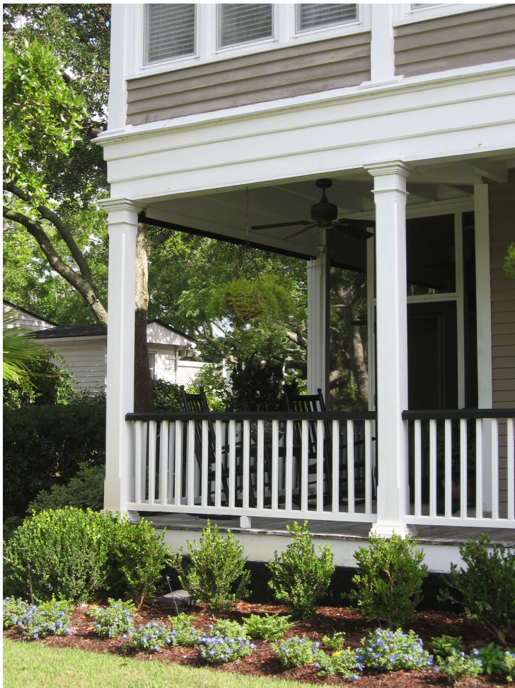
Home owners can familiarize themselves with the principles of appropriate treatment of historic features such as the repair of original chamfered wood columns and balusters (1722 Middle Street).
