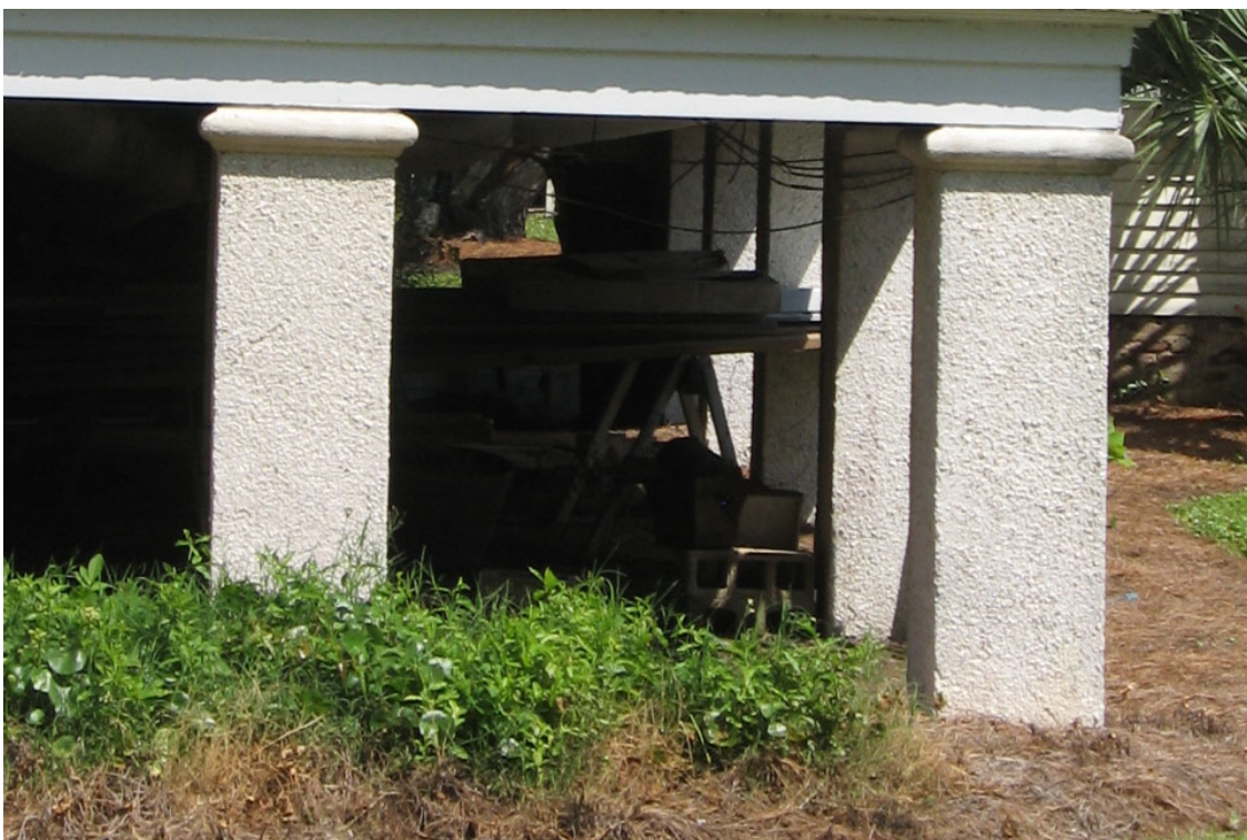
Foundation piers for dwellings are often of concrete and stucco materials such as at 1820 Middle Street.
